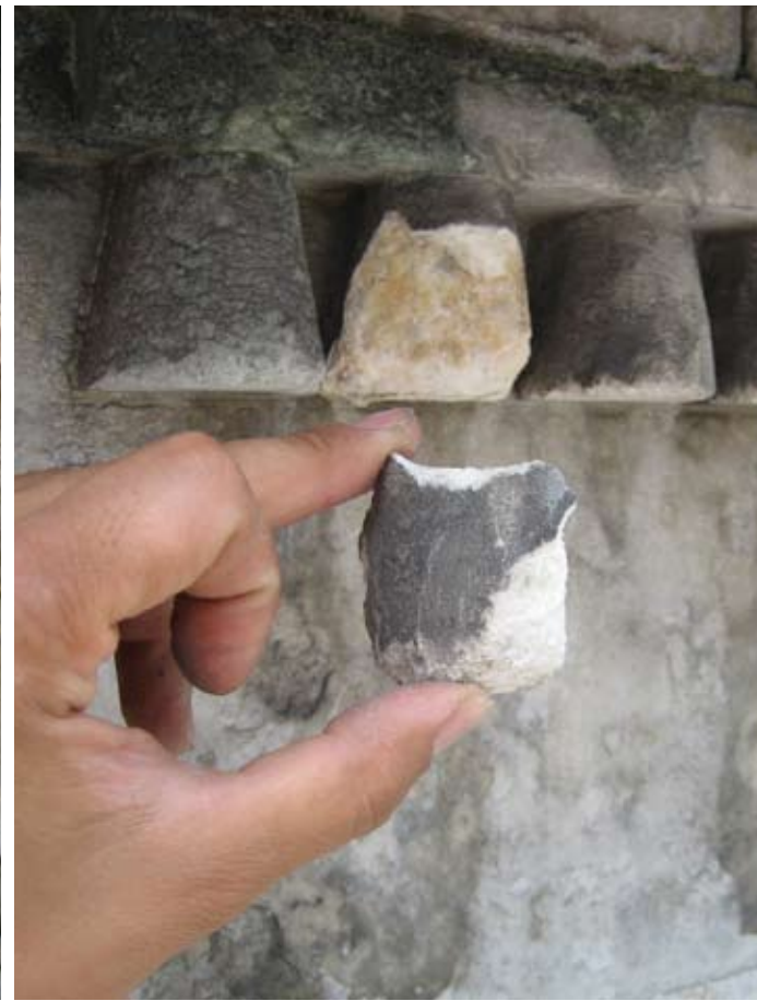
Pieces of the Humanities and Social Sciences Library that were in danger of falling were removed for repair.
